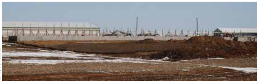
Pictured above is the construction of West View 4, an individual bull housing barn for EU qualified sires in-waiting. This building project along with the new EU Isolation Barn and new Feed Station are scheduled to be completed by mid-summer 2008.
